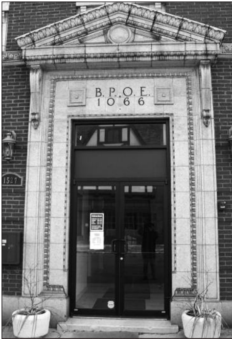
The exterior of the Elks Building has been restored, and all of the ornamental terra cotta has been repaired and cleaned.
